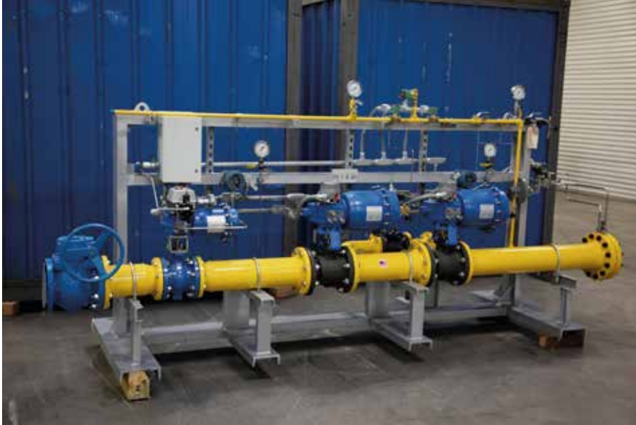
Fuel Piping Module
