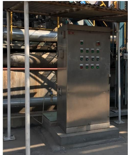
Typical NTFB BMS/CCS Panel
