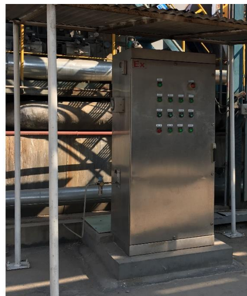
BMS - Nema 7 Explosion Proof S.S. Remote Burner Light off Panel
